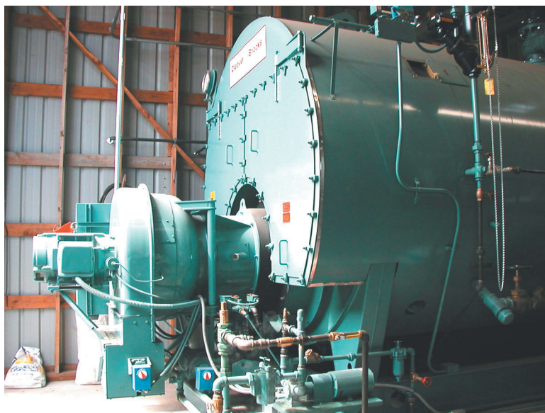
Steam generator inside building containing distilling apparatus
